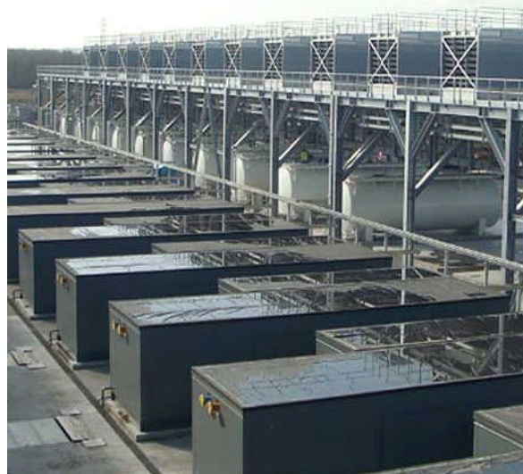
The equipment yard at Google's chillerless data center in Belgium
